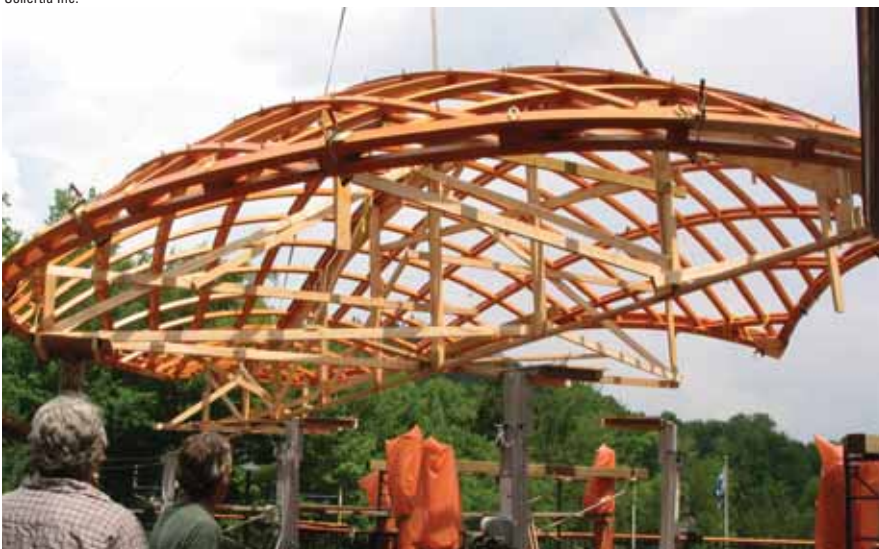
The 50-foot-long structure is moved by crane from the workshop to its final destination.
