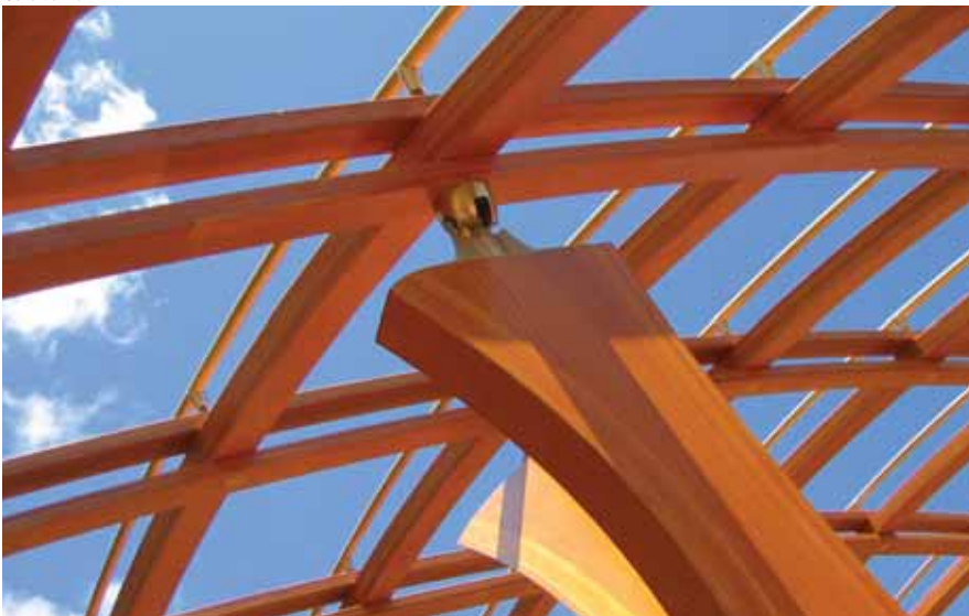
Most of the painstaking woodworking for the structure involved laminated double curves.
